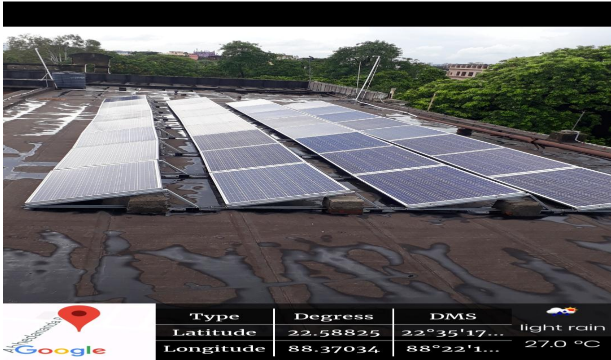
Fig B: Solar panels on roof top
