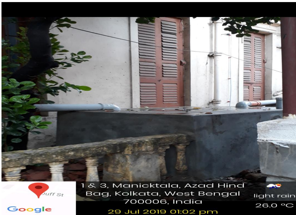
Fig E:Reservoir of roof water harvesting
